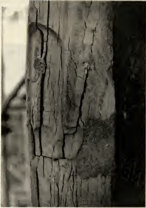
Fig. 20. Vertical cracking along bedding planes of tuff at intersection of east wall of nave and transept. Cementitious mortar repair in areas of loss (Photo: Anne Brackin).
